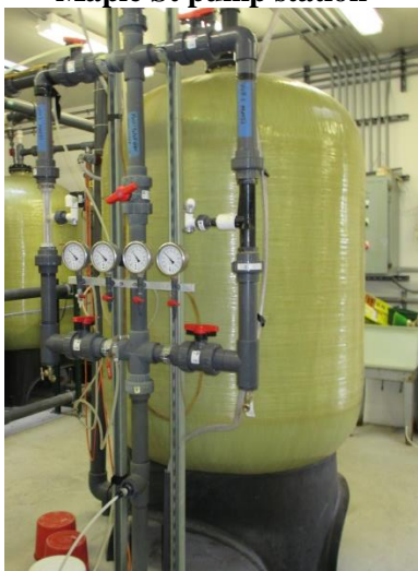
Two mazzes for air suction, prechlorine injection point shown at the bottom
