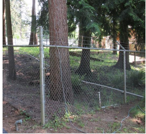
Bachwash water sprinklers
