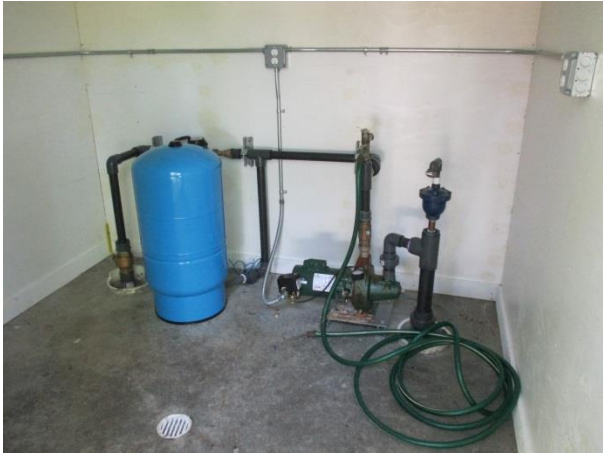
Maple St pump station
