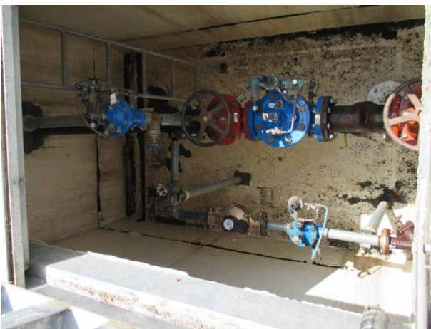
PRV vault at Driftwood
