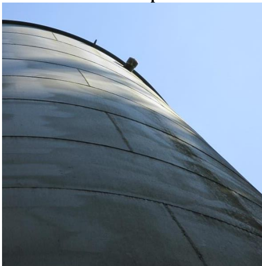
300K reservoir, rusted and worn outside
