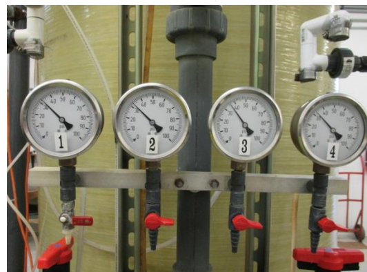
pressure gauges for the treatment
